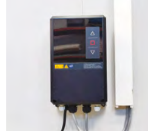
Centralina Control Panel
